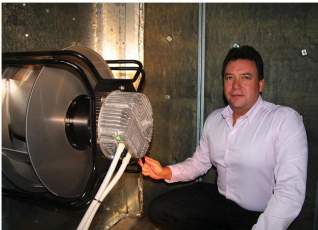
Figure 3: Kevin O'Reilly (System Solutions Engineering) with a new ebm-papst EC plug fan in one of the building's air handling units.
