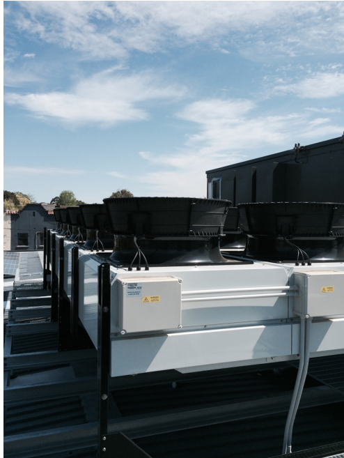
Figure 1: ebm-papst EC fans on top of the Bocaccio Cellars roof
