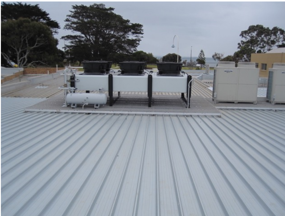
Figure 1: The installed rooftop unit at IGA San Remo
