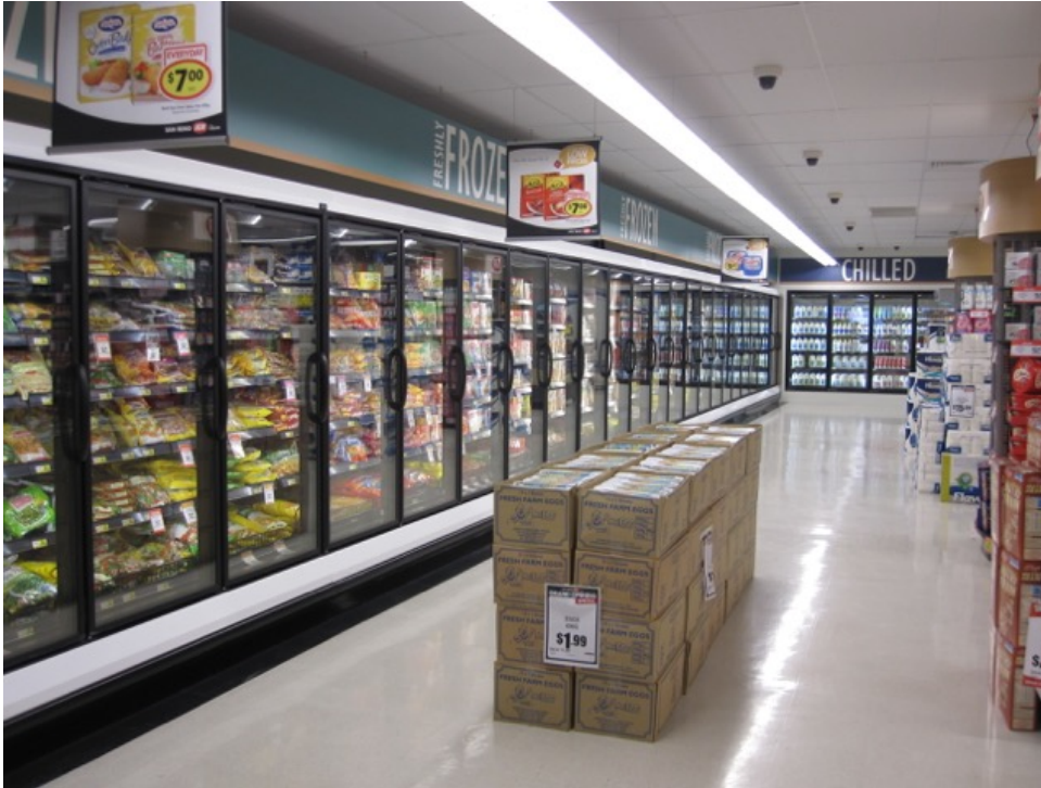
Figure 2: New efficient fridge cases fitted with ebm-papst EC motors
